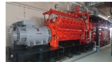
Energy Center (Standby Generator)
