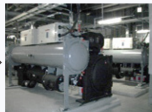
Turbo-type refrigeration unit powered by electricity
